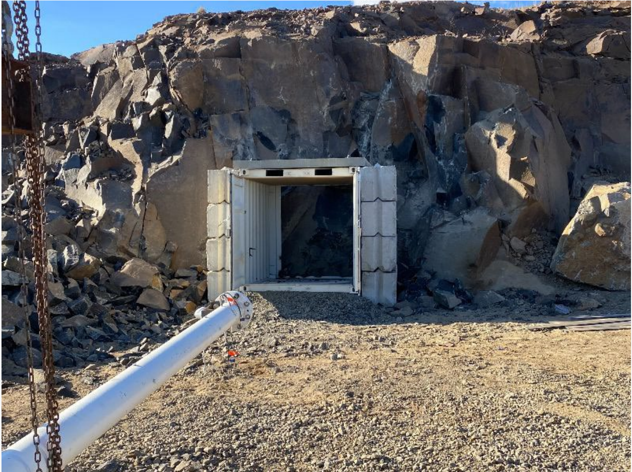
Figure 1: The tunnel begins! Hyper tunneling demo now has 2 major mining partners participating!
