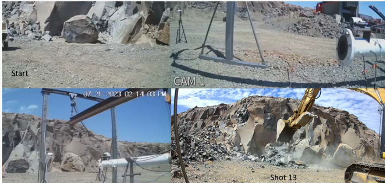
Figure 2) Boulder Buster!!! HyperSciences successful commission and integration of the first HyperDrill™-HyperBreaker™ full test kit at site and testing in the tunneling field trials. Customer-requested boulder busting demo (Click picture or HERE for video). Fueled by clean hydrogen and/or propane (Planned Future: Biodiesel).
